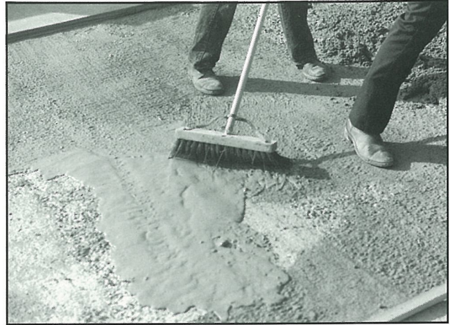
Fig. 1. Just prior to placing the concrete topping mix, broom a grout into the surface to provide a bonding course between the old and new surfaces.
